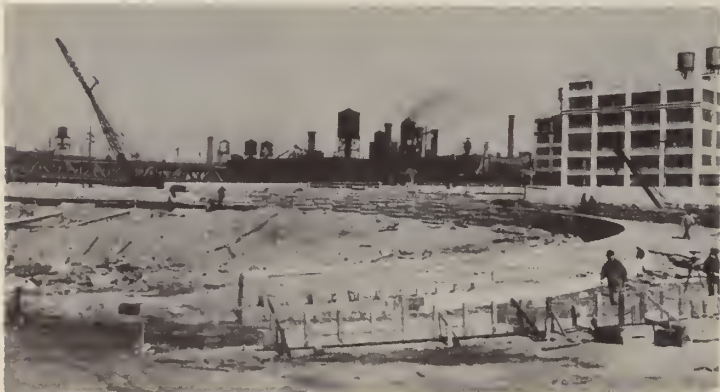
The new exit for the south roadway into Fulton Street takes shape.
